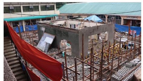
The City Government of Bago embarks with the construction of the 2- storey Jubilee Hall Building at the Bago City Hall compound last October 19.
